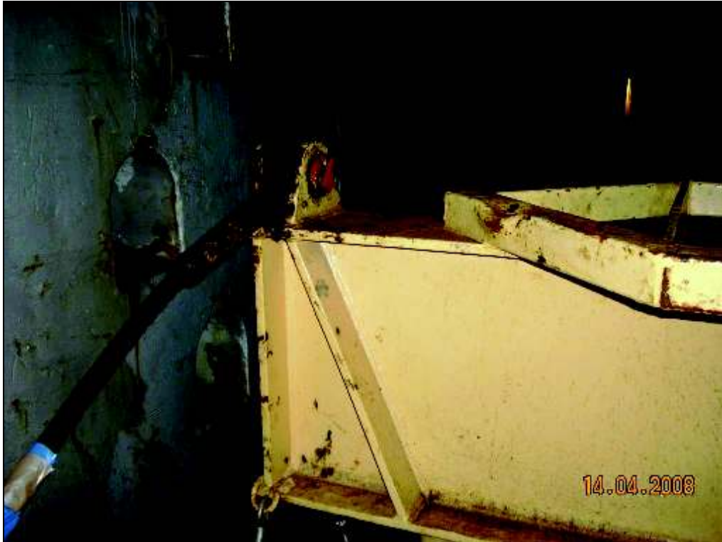
Figure 4. View of hoist wire connection at one end of the tween deck lifting beam
