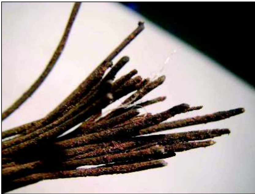
Figure 6. Wire breaks at an outer strand at the point of failure of the wire.
