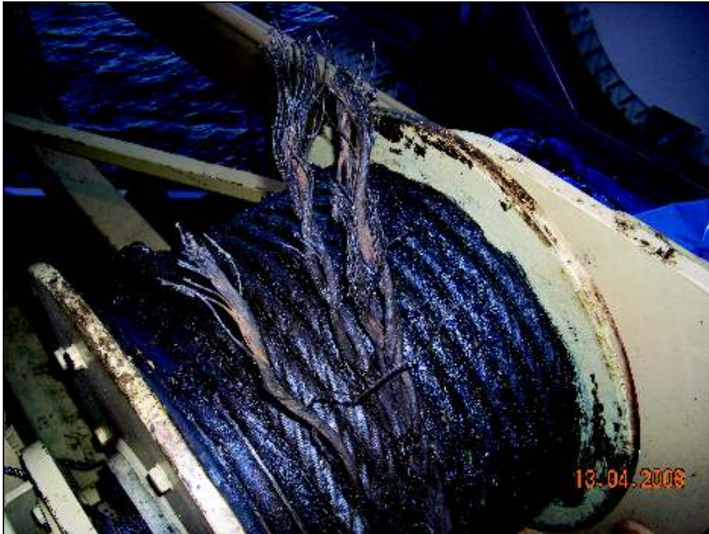
Figure 5. View of failed hoist wire at winch drum showing level of greasing present on wire during normal operation. Corrosion product is also visible on the de-stranded wires at the point of break.
